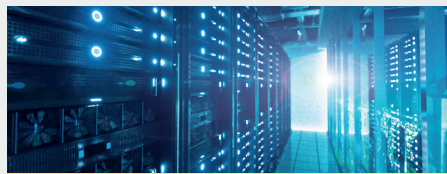
Emergency power/UPS systems
